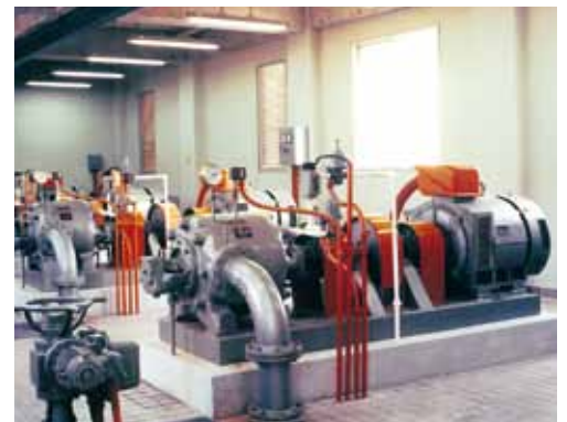
Distributing pumps in small-capacity water works
